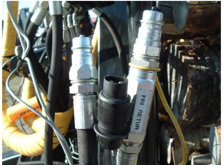
Hydraulic and electrical connections for crane and support legs (on a trailer with lightweight package).
